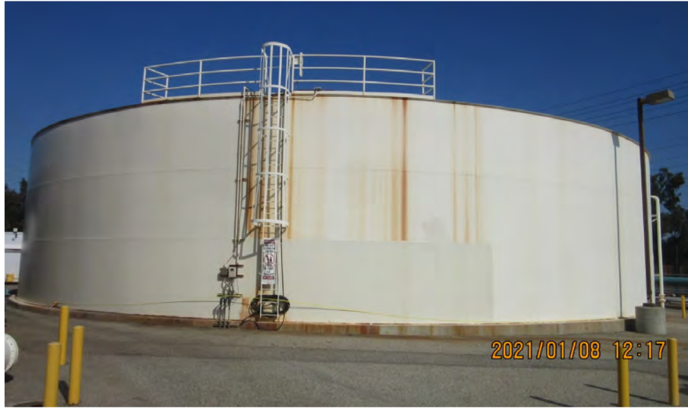
700,000-gal steel nitrified product water storage tank at TRWRP
