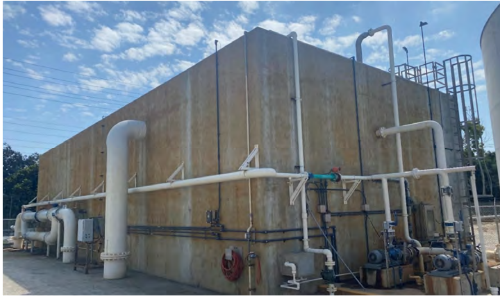
Waste Discharge Basin at TRWRP
