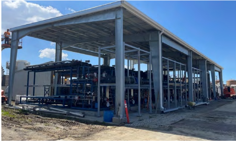
Custom Engineered Microfiltration System at JMMCRWRP
