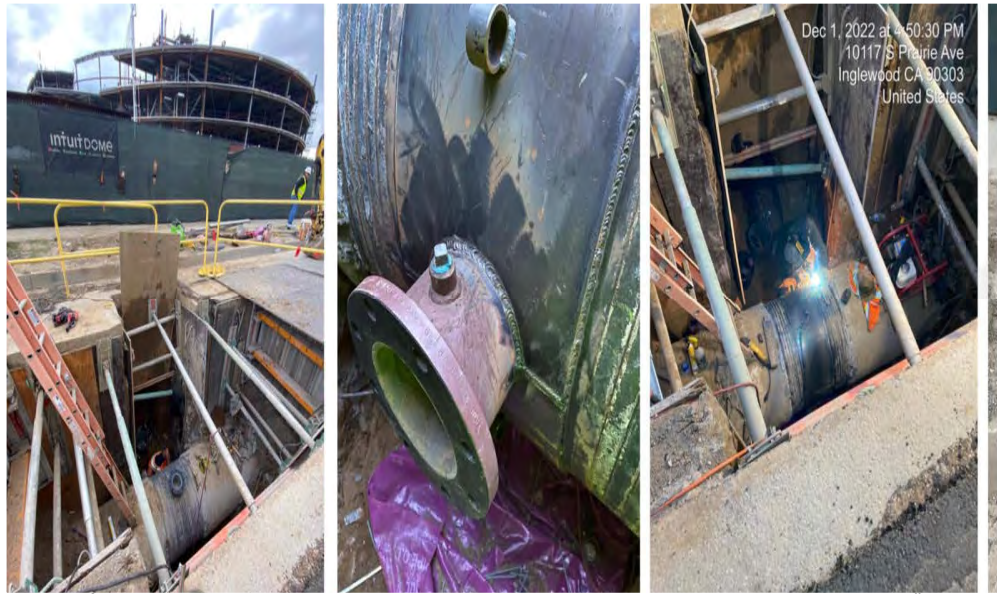
Left photo to Right photo: Project Site, 6-inch welded Nozzle outlet, Welded Wrapper Plate onto 36" existing pipeline
