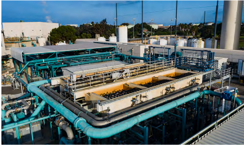
Microfiltration Membrane System at ECLWRF
