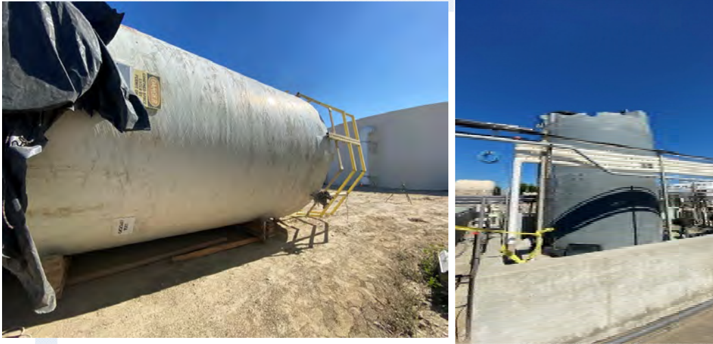
Right photo: SHC tank out of service. Left Photo: Temporary SHC tank.
